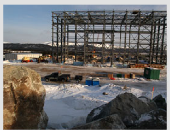
Structural steel in place for concentrator building at Voisey's Bay construction site.
